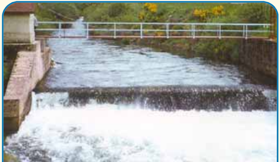
A weir of the scale envisaged at Eastgate as part of the proposed hydro-electric power scheme
