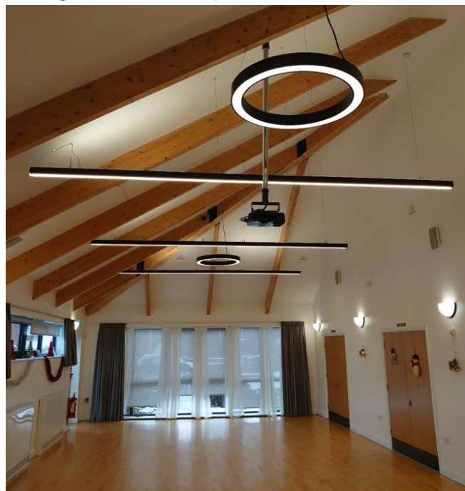
The new energy efficient LED lighting scheme
