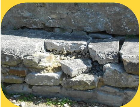
A vandalised wall seat adjacent to The Manor pub.
