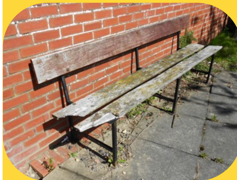
Dilapidated bench in Dorset Place.
